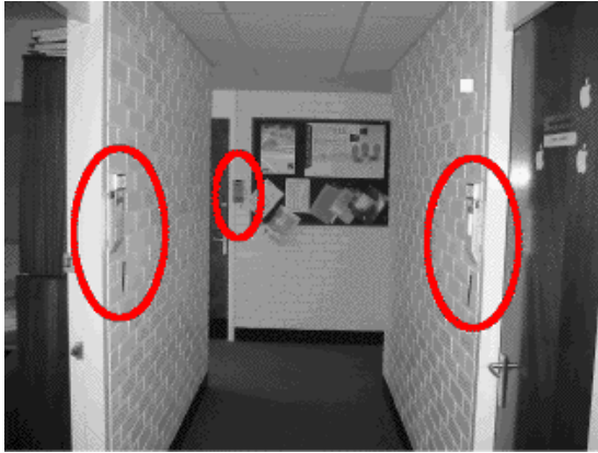
Hermes units in the corridor
